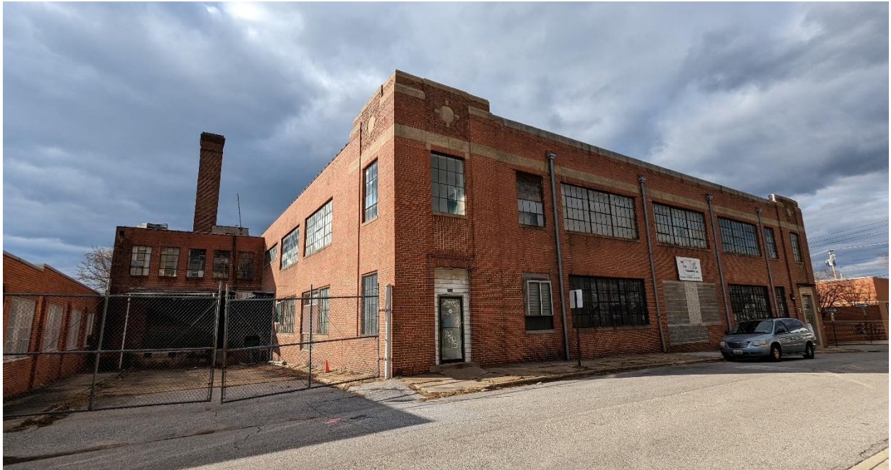
Image 18: The East elevation faces Elm Avenue. The chimney stack, while set back from the street, is a prominent feature of the building.
